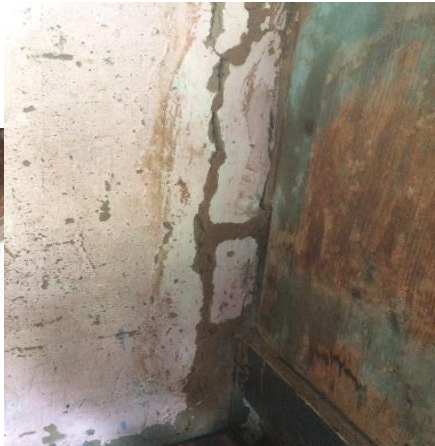
Cracks due to corner
